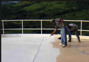
Water Tanks - Honduras
