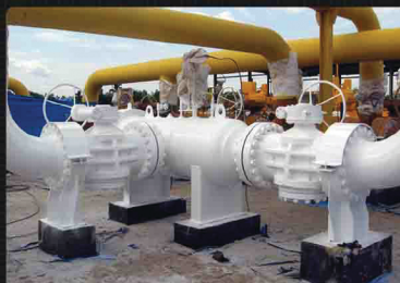
Gas Pipeline - Indonesia
