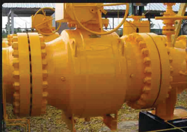
Gas Pipeline - Indonesia
