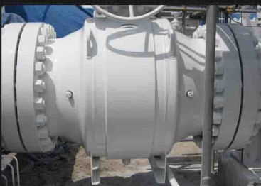
Gas Pipeline - Indonesia
