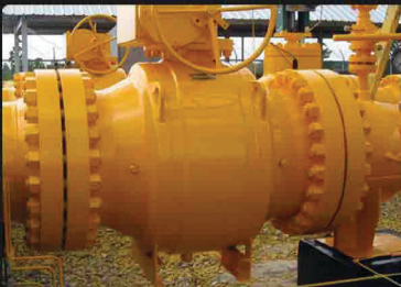
Gas Rohr - Indonesia
