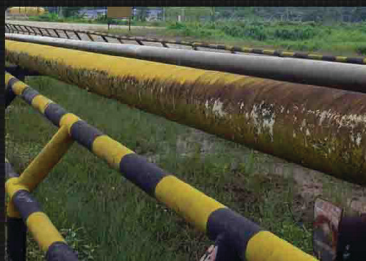
Gas Rohr - Indonesia
