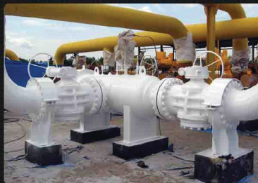
Gas Rohr - Indonesia
