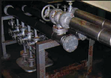
Steam Pipes - Turkey [before]
