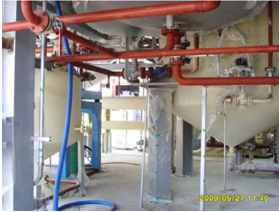
<Tank and Condenser>
